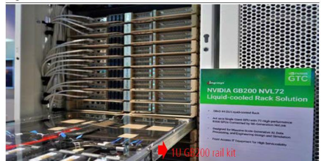
Figure 24: Server rail kit in an NVL72 rack
