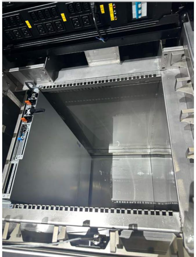
Figure 43: Immersion cooling tank interior
