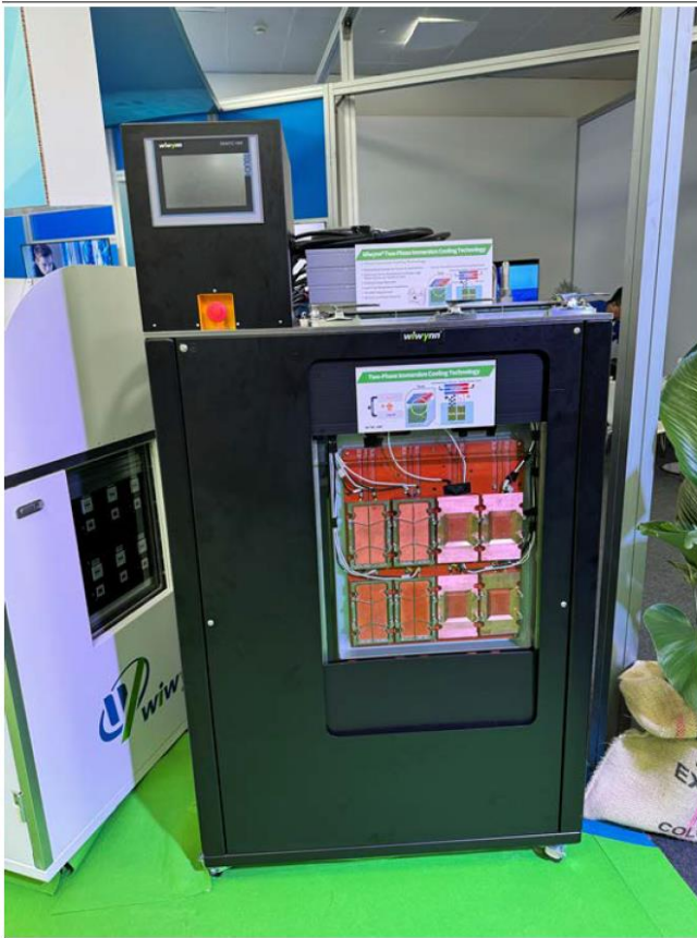
Figure 34: Wiwynn's two-phase immersion tank
