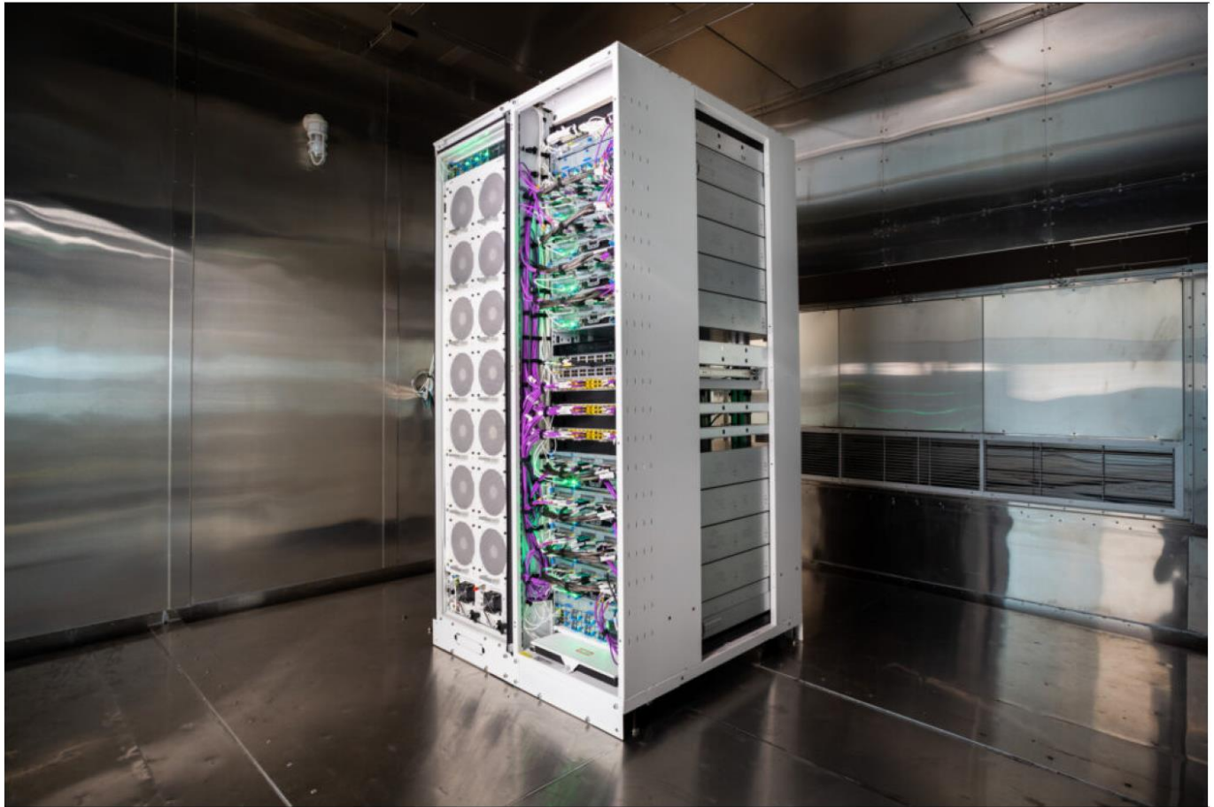
Figure 5: AEC (purple cables) are used in Microsoft's Maia server rack
